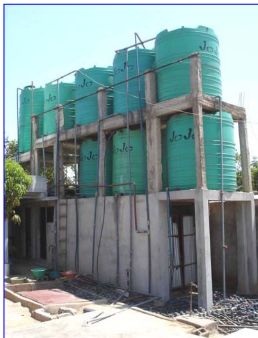
Photo 1: Private storage tanks in Maputo (Mozambique)
