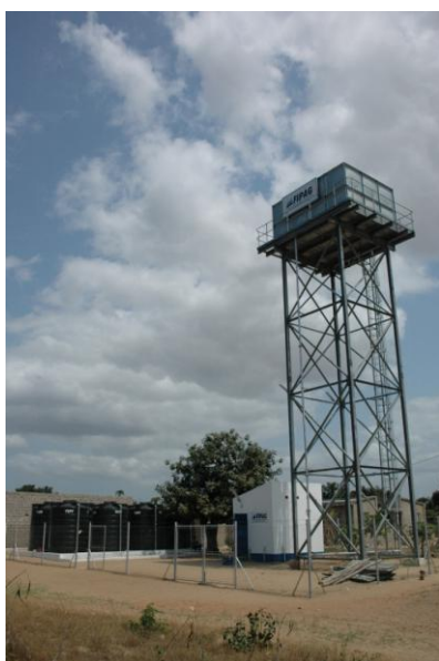
Photograph 3. “FIPAG” system in Zimpeto
